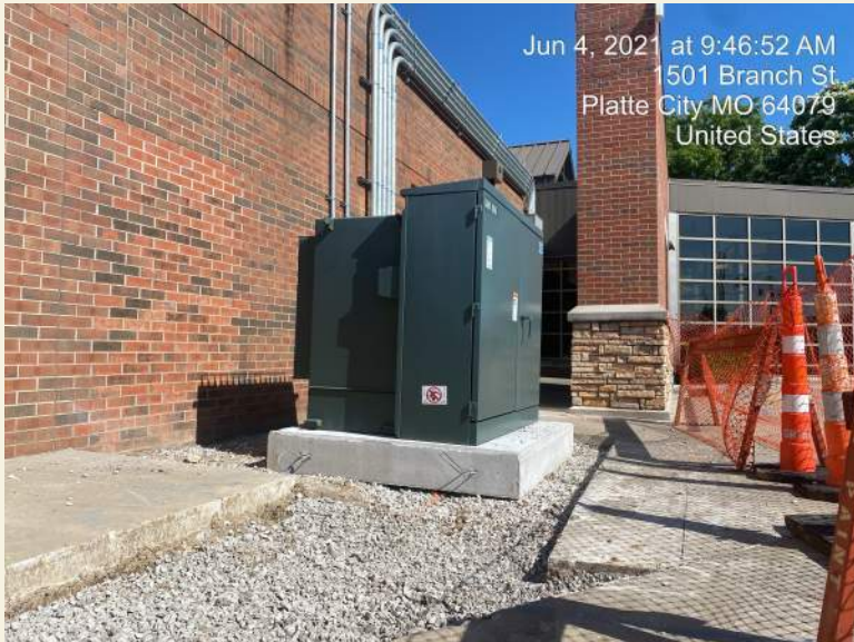
Transformer relocated to East Side of Building
